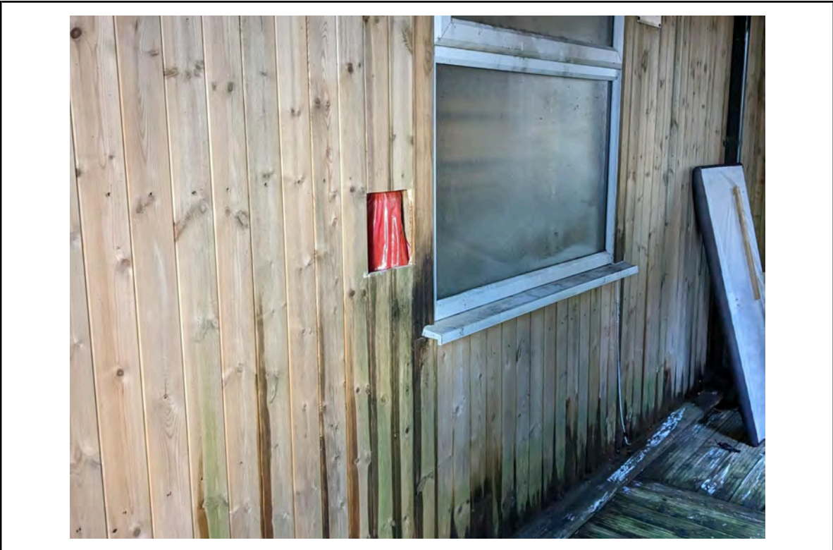
Photo 49: Location 23 - Timber cladding removed on 1st floor at inner courtyard elevation
