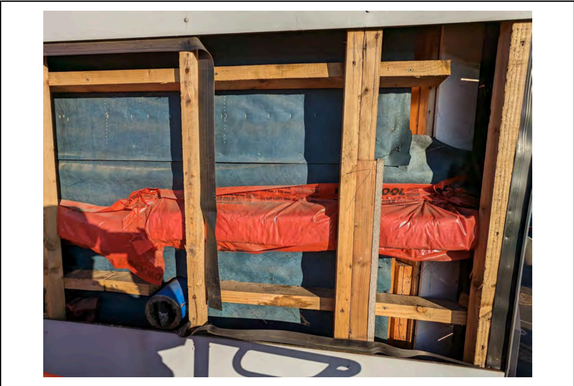
Photo 17: Location 7 - HPL removed on 3rd floor at south elevation
