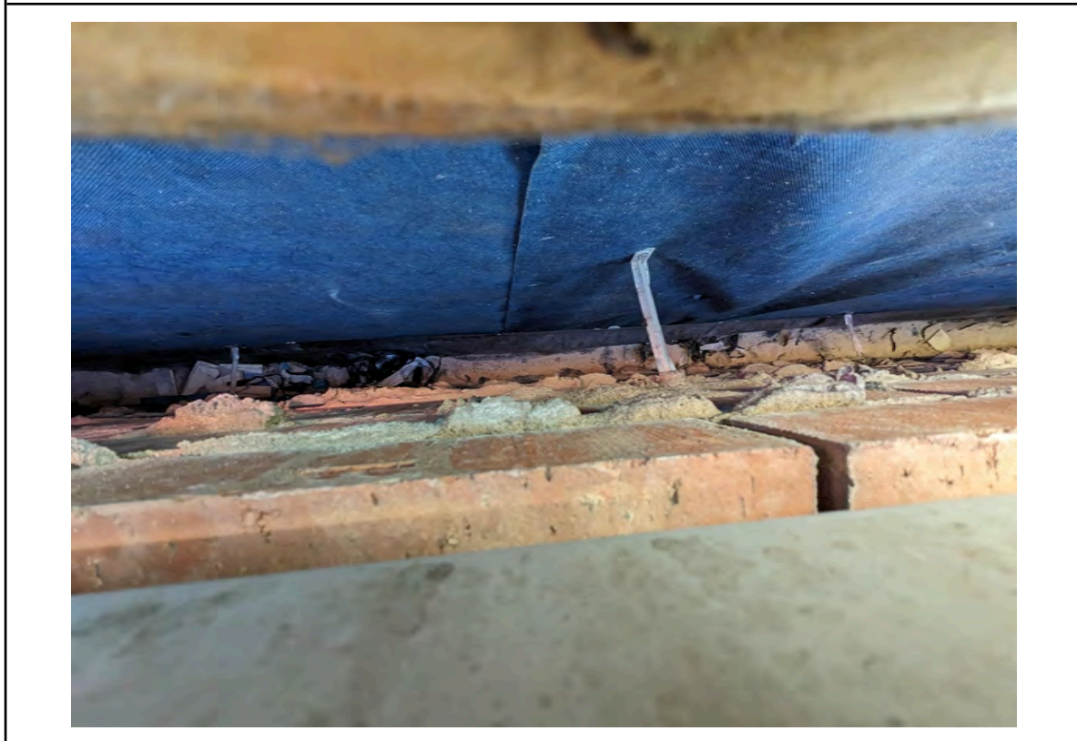
Photo 6: Location 1 - Cavity showing absence of horizontal barriers at compartment floors
