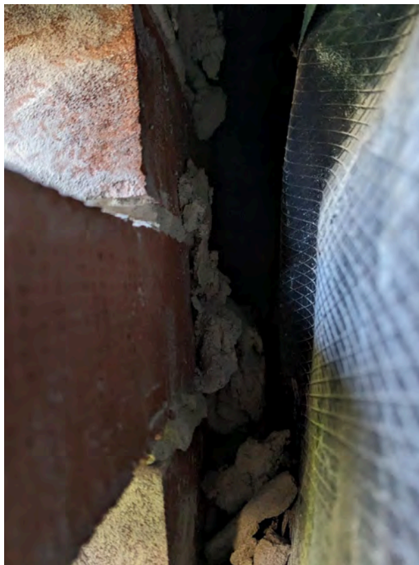
Photo 60: Location 28 - Cavity with no cavity barriers in line with compartment walls and floors
