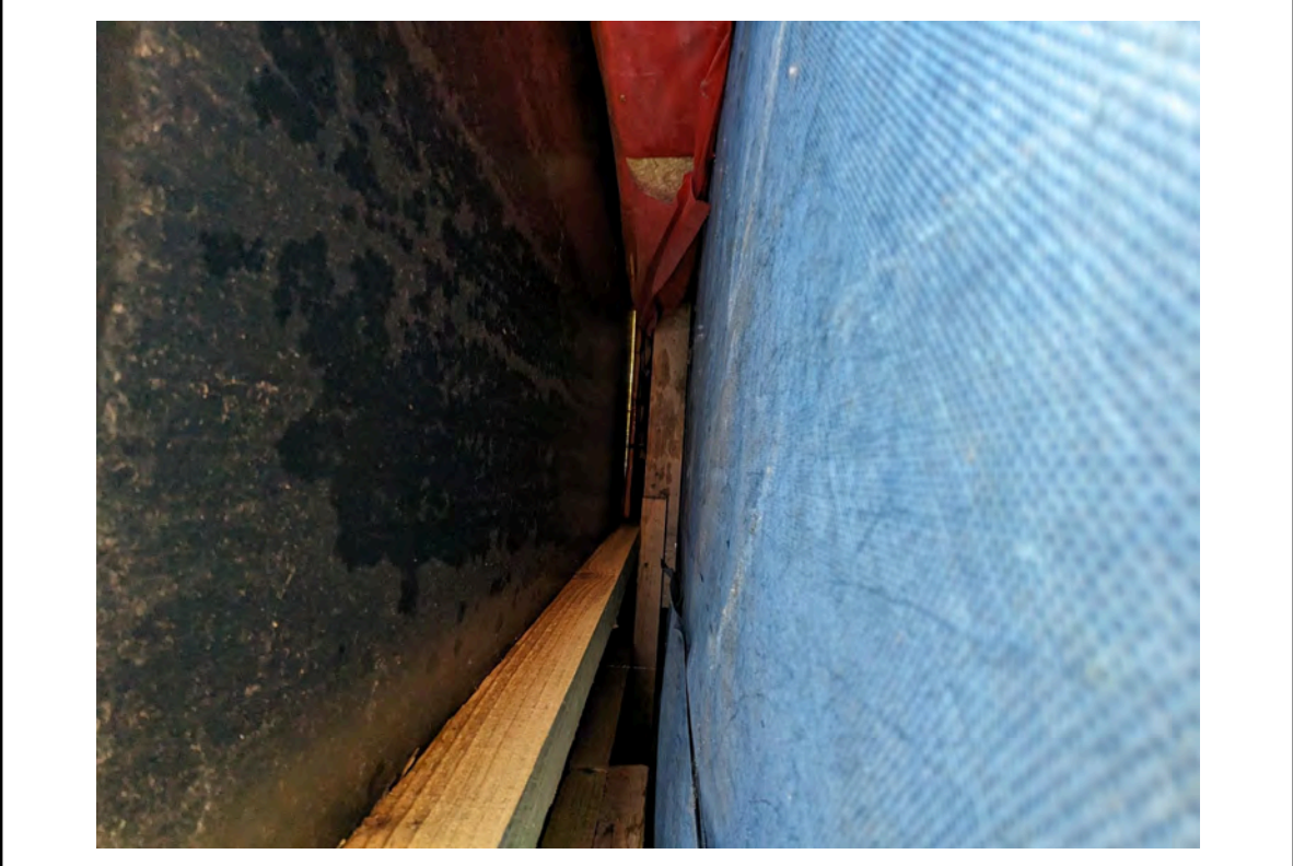
Photo 28: Location 12 - Cavity showing the timber studs, breather membrane and horizontal barriers, but no vertical barrier
