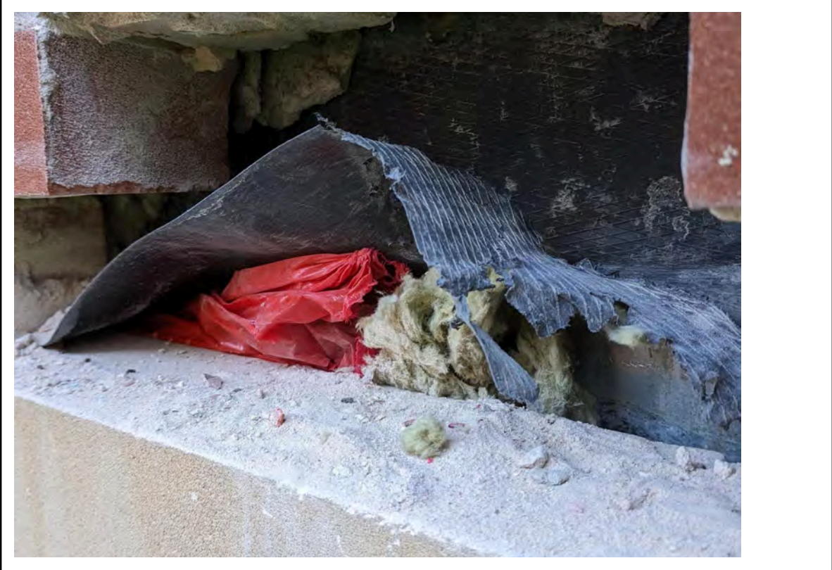
Photo 42: Location 19 - Cavity showing the cavity barrier, cavity tray, breather membrane and wall ties
