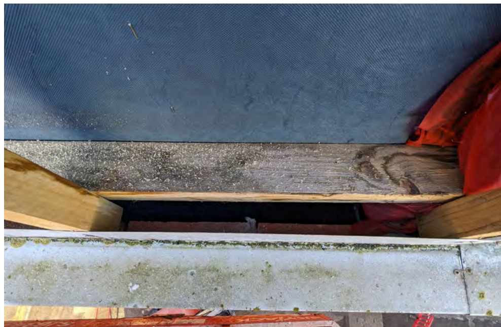
Photo 38: Location 17 - Cavity showing the cavity barrier at window openings, but no horizontal barrier between floors
