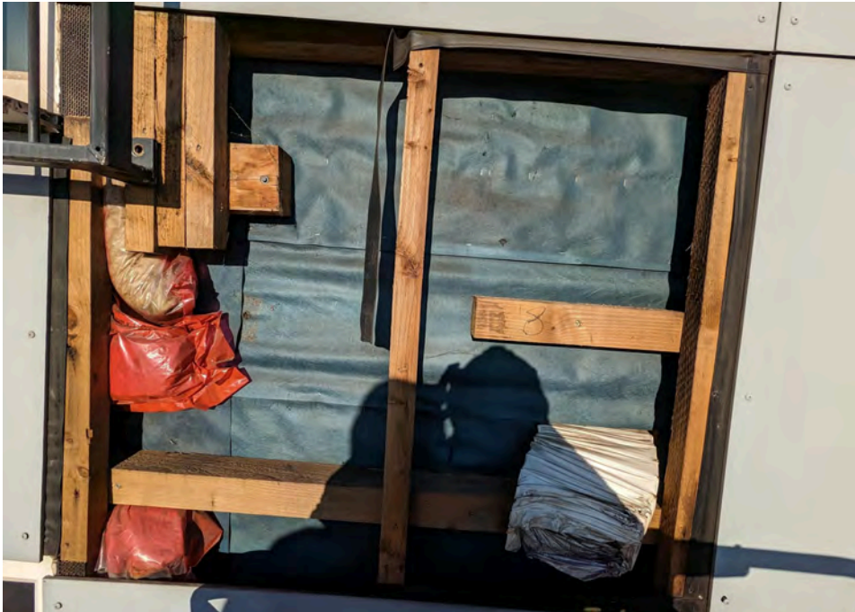
Photo 19: Location 8 - HPL removed on 3rd floor at south elevation
