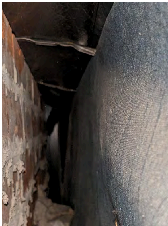
Photo 22: Location 9 - Cavity with wall ties, breather membrane and damp proof membrane and barriers
