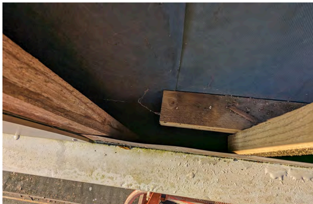
Photo 30: Location 13 - Cavity with timber studs, breather membrane and vertical barriers, but no horizontal barrier between floors.
