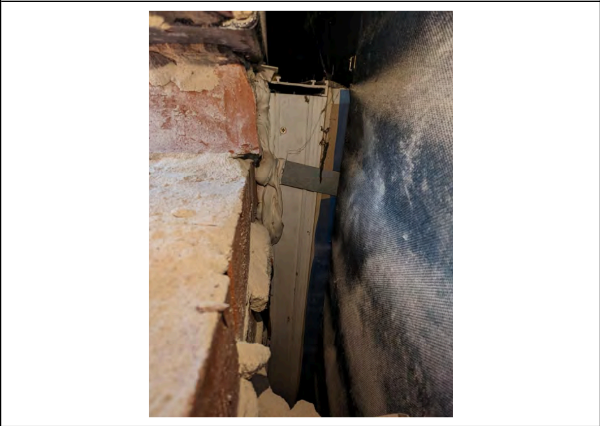
Photo 8: Location 2 - Cavity with wall ties and breather membrane, but no cavity closer at window opening
