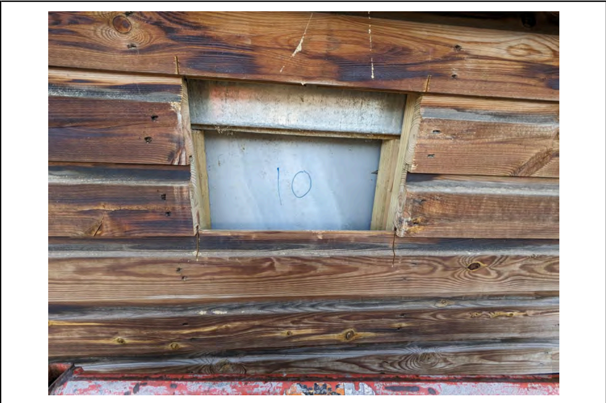
Photo 23: Location 10 - timber spandrel panel cored out on 1st floor balcony at business centre entrance
