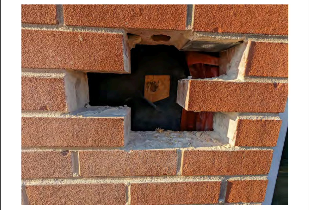
Photo 32: Location 14 - Brick build up
