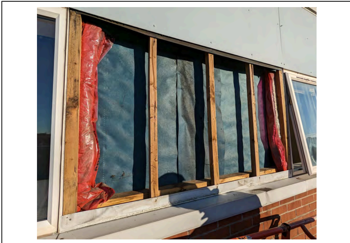
Photo 5: Location 1 - HPL removed on 3rd floor on 3rd floor at South West Elevation
