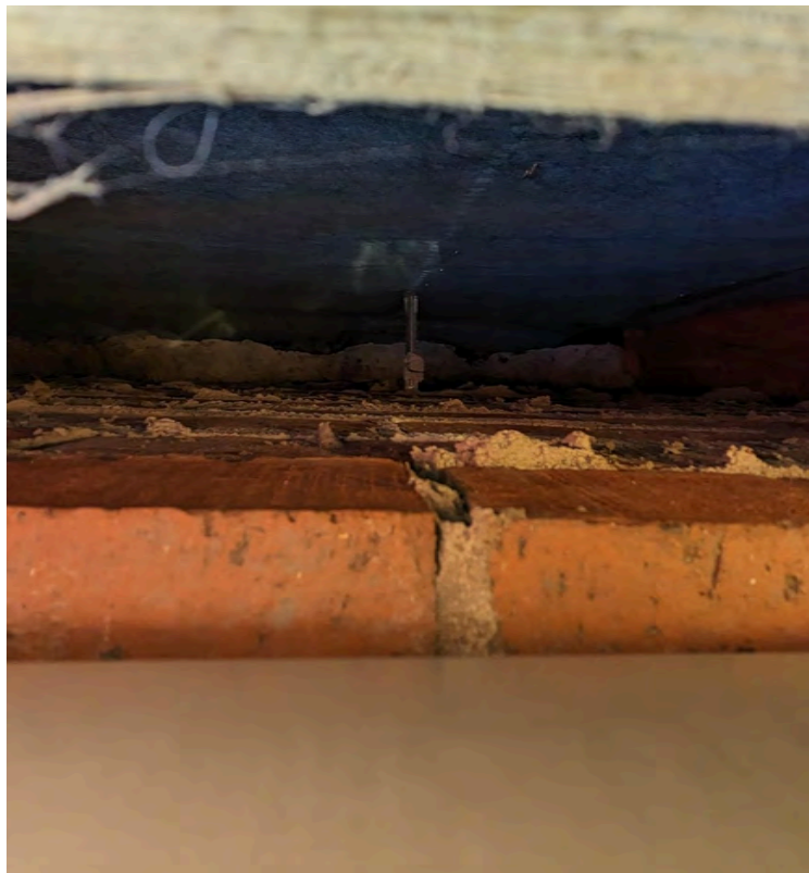
Photo 36: Location 16 - Cavity with breather membrane, wall ties, cavity closer, but no cavity barriers.
