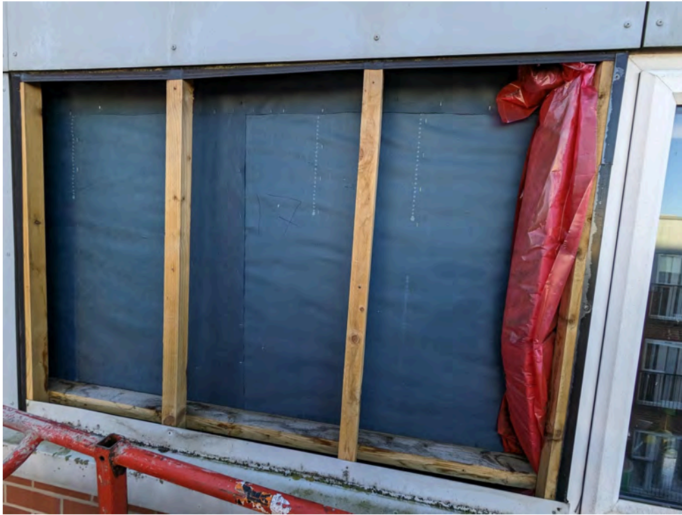
Photo 37: Location 17 - HPL removed on 3rd floor at north elevation
