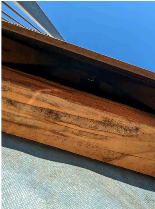
Photo 20: Location 8 - Cavity with timber studs and breather membrane, no horizontal barriers between compartment floors
