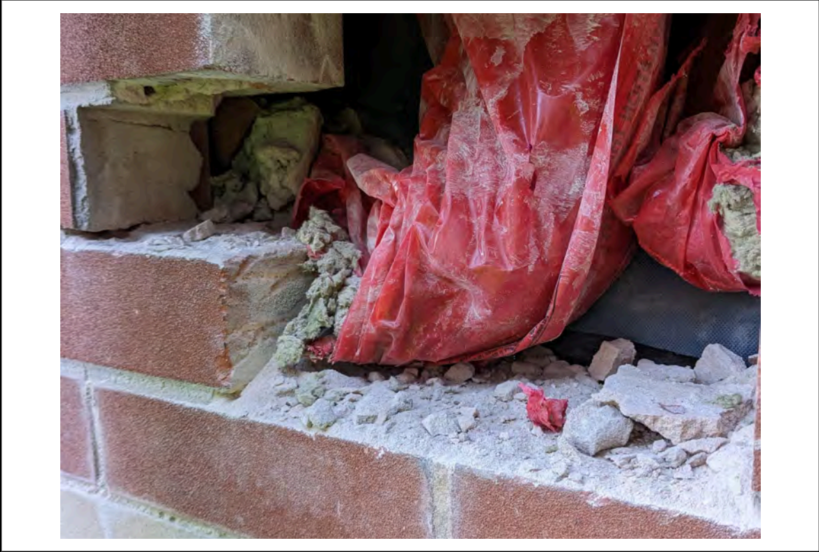
Photo 44: Location 20 - Cavity showing the cavity barrier, cavity tray, breather membrane and wall ties
