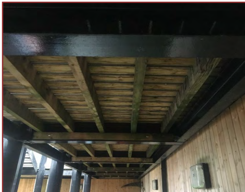
The timber decking of the walkways in the inner courtyard shown from below with softwood timber joists.
