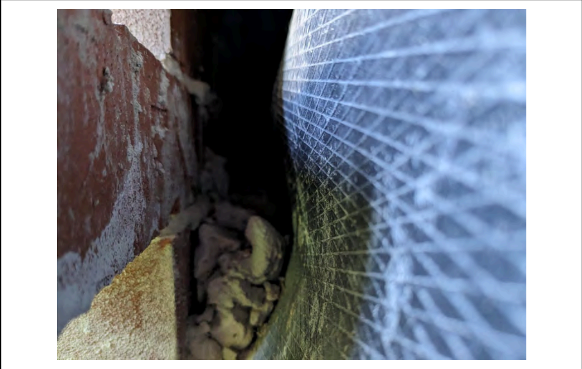
Photo 64: Location 29 - Cavity with no cavity barriers in line with compartment walls
