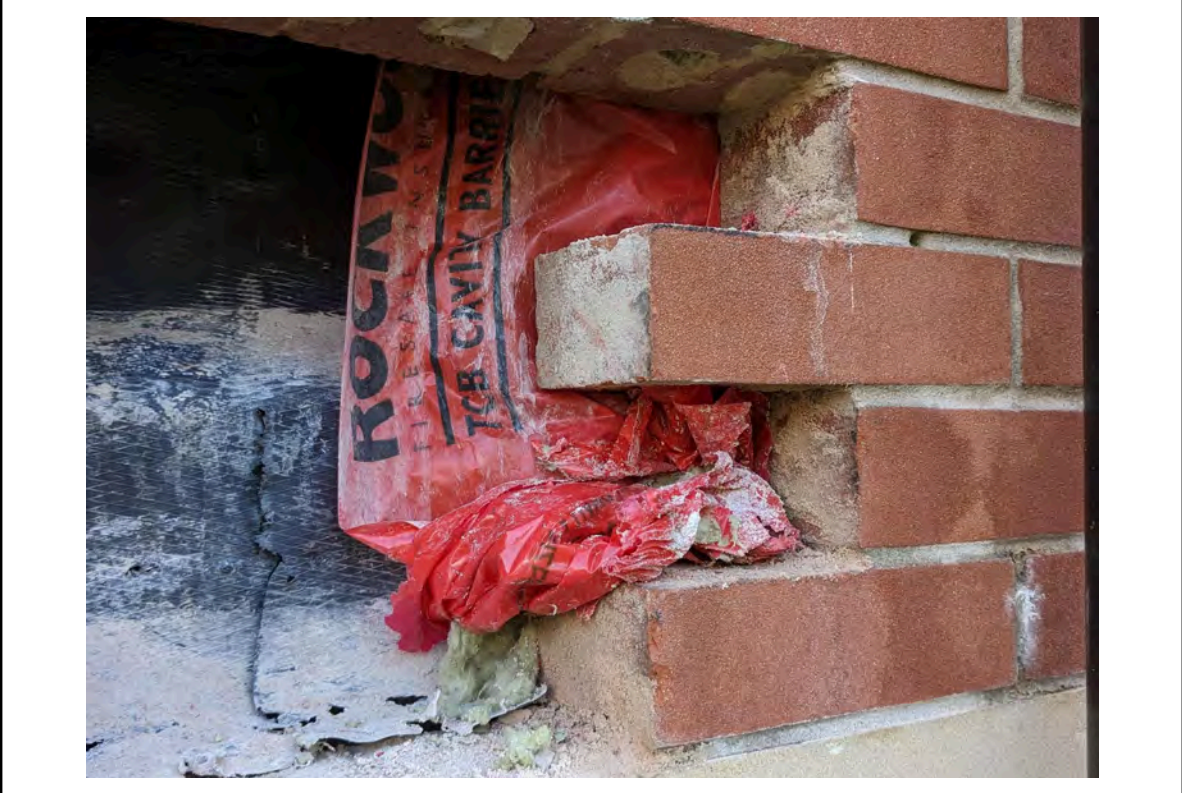
Photo 40: Location 18 - Cavity showing the cavity barrier, cavity tray, breather membrane and wall ties
