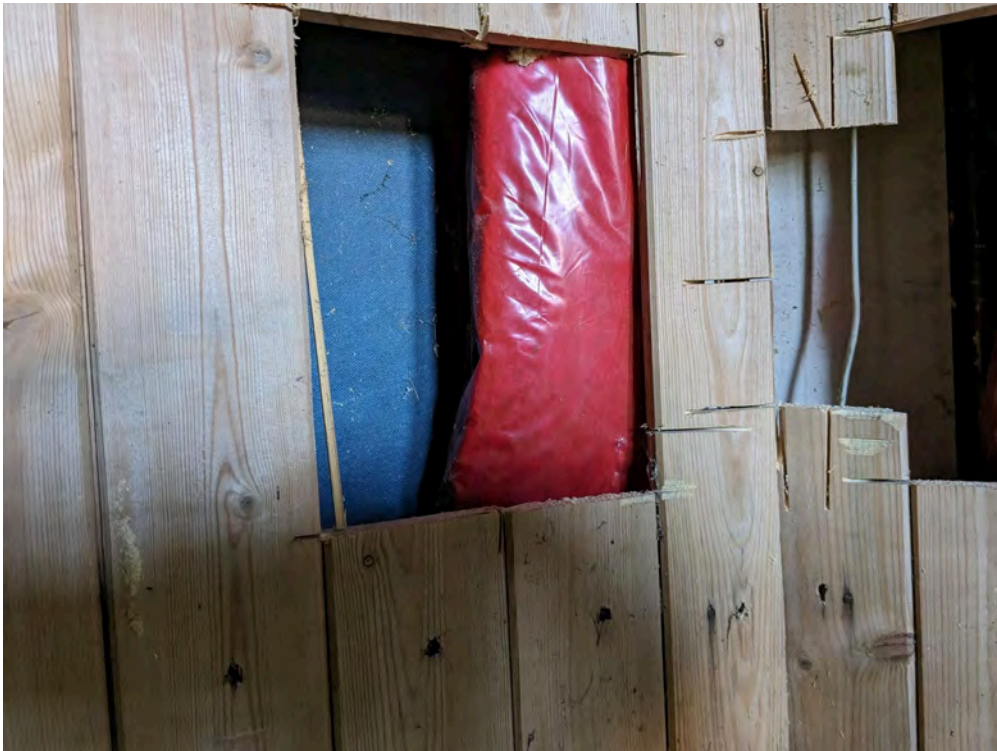
Photo 52: Location 24 - Cavity with vertical barriers, breather membrane and electric wiring with thermoplastic insulation
