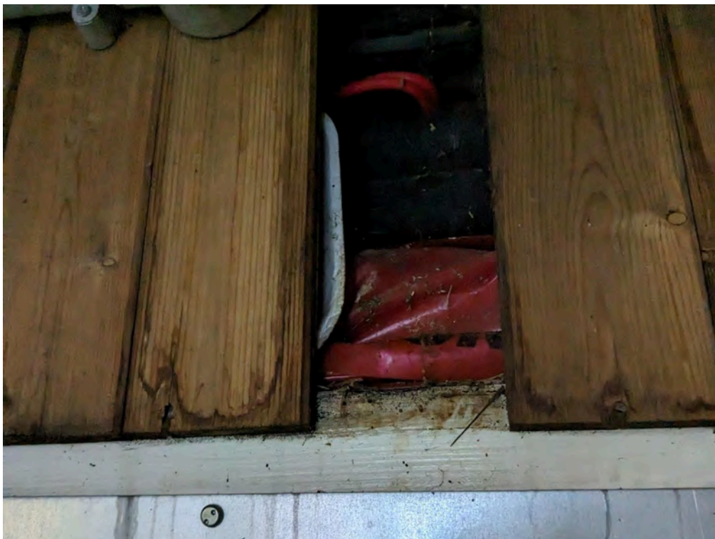
Photo 56: Location 26 - Cavity with cavity closers at door openings, thermoplastic insulations and breather membrane
