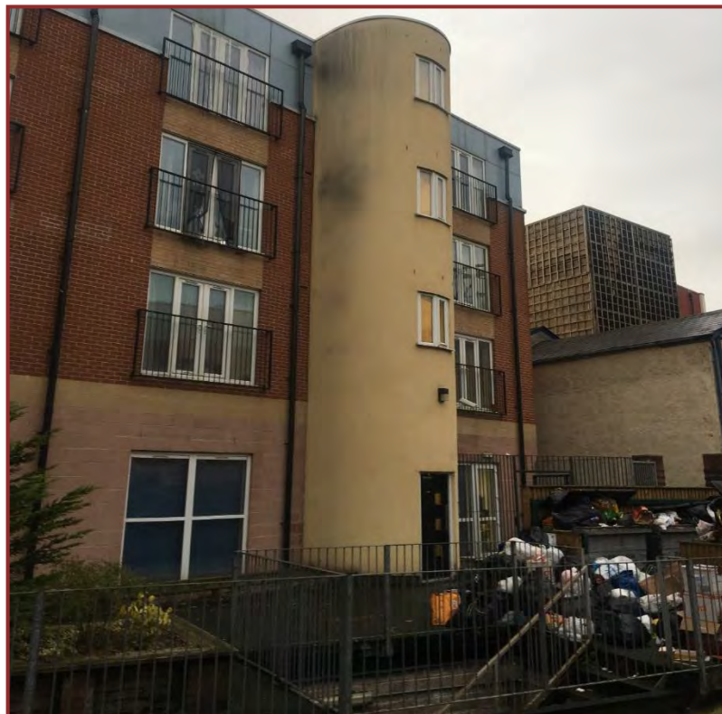
The rear courtyard contained rendered columns with curtain walling to the ground floor commercial space and ground to floor feature area windows to each flat with Juliette balconies.
