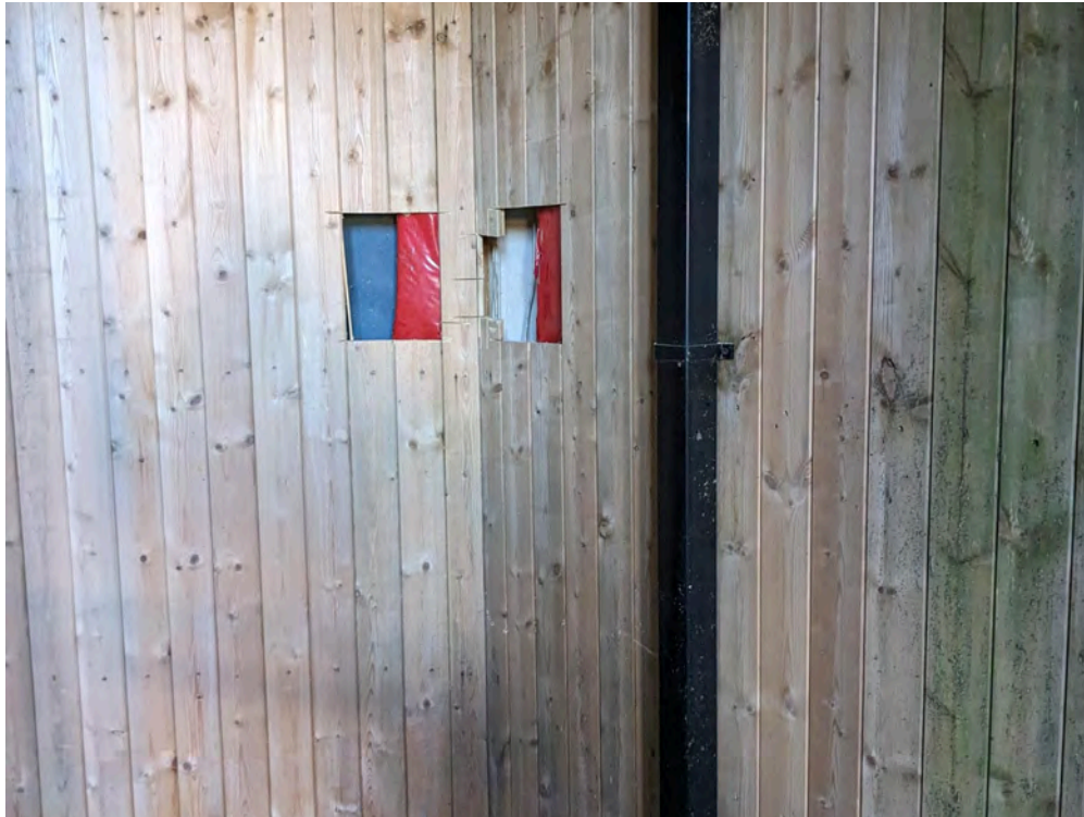
Photo 51: Location 24 - ETICS cored out on 1st floor at side elevation
