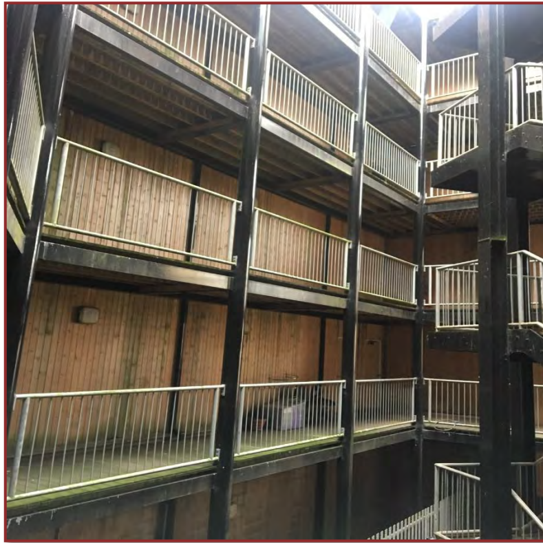
Inner courtyard area clad in timber with doors to each flat and a central staircase with access to the flats.
