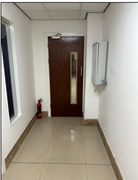
Internal Fire Door Example
